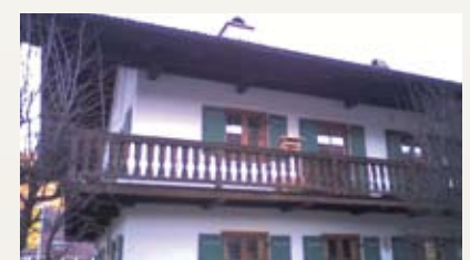
Bad insulation above balcony window
