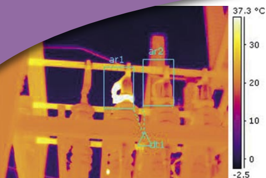
Hot spot at substation: urgent repair
