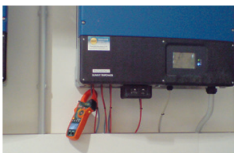
These inverters convert the direct current from the solar panels to alternating current.
