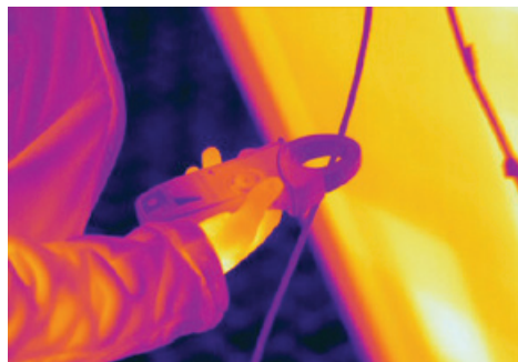
The amount of electricity the panel produces can quite easily be measured with the clamp meter. The measurement data are combined with the thermal image with the help of FLIR MeterLink technology.
