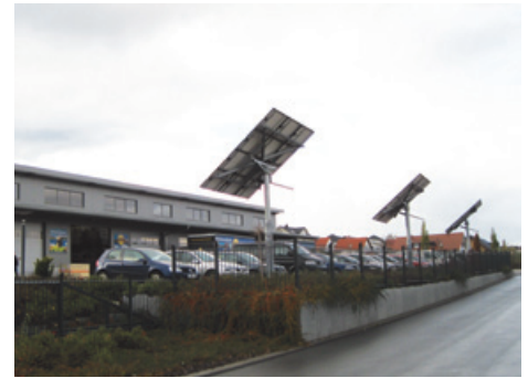
These solar panels that are mounted on poles can be scanned from the back to minimize reflection.
