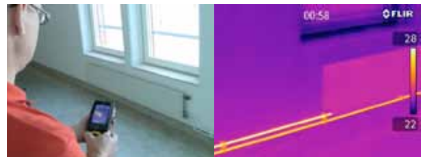
The radiator in the thermal image is clearly not functioning well. The hot water pipe is probably clogged.
