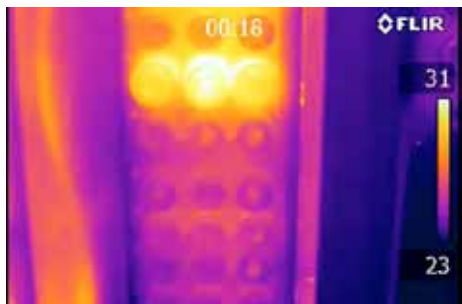
Where a spot pyrometer shows the temperature in one area, a thermal imaging camera can give an overview of an entire electrical cabinet, enabling quick and accurate faults detection.
