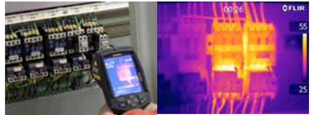
The thermal image clearly shows which fuses are too warm and will soon need to be replaced.
