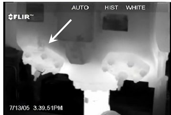
Figure 10, LPG compressor flange leak, darker area just off arrow tip.
