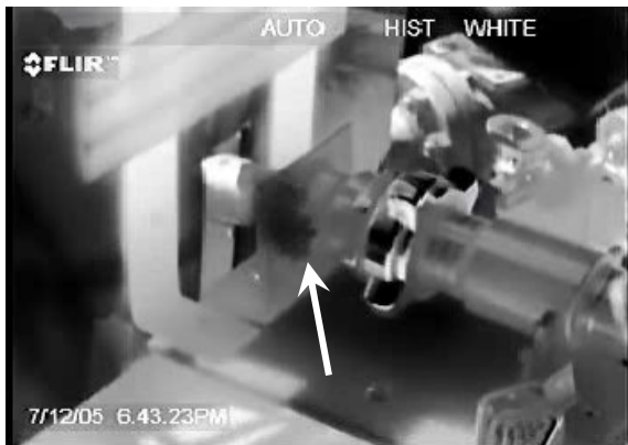
Figure 9, LPG pumping station transfer line leak, dark cloud just above arrow.
