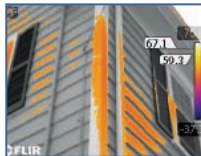
Moisture located on siding and wooden trim of house.
