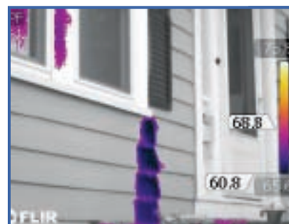
Window sill leak noticeable from exterior of house.
