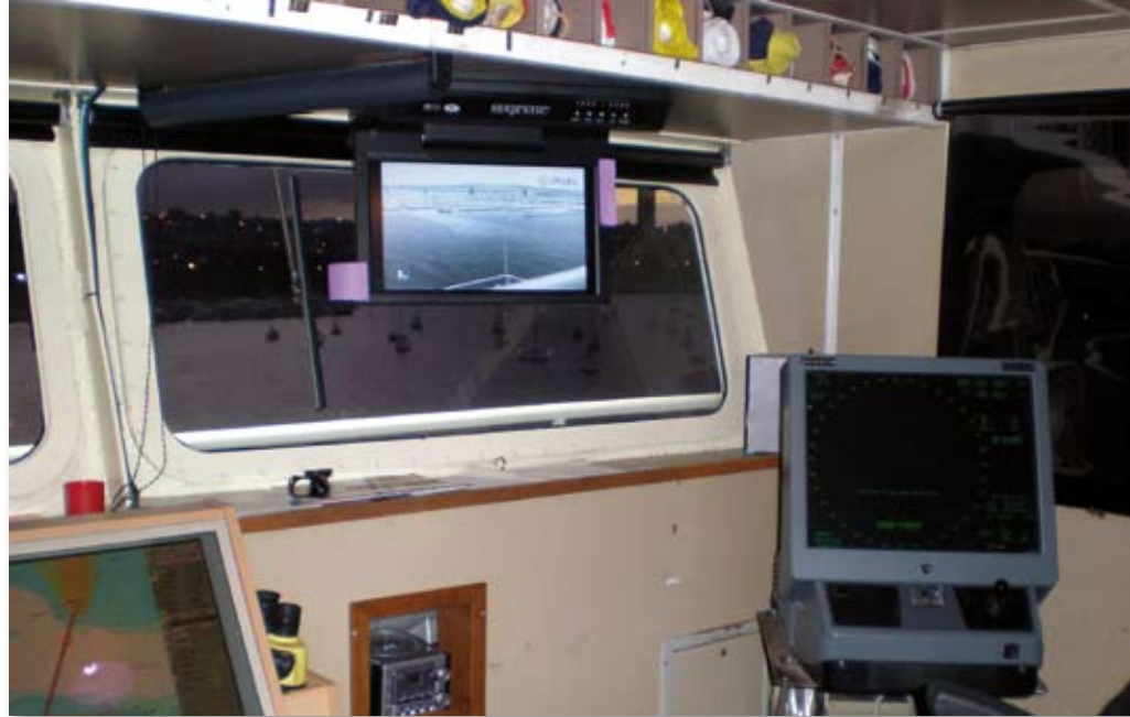
The FLIR Systems Navigator produces a crisp image which is projected on a 20" LCD screen installed on the bridge.
