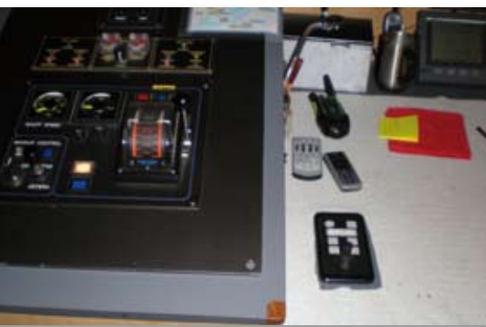
The Joystick Control Unit for the Navigator Pan / Tilt is integrated in the bridge.
