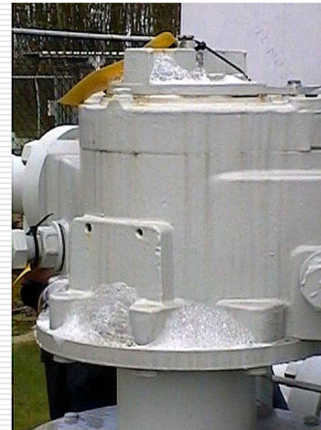
Figure 2.1. Bubble test on leaking valve
